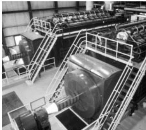
Installation de cogénération © UIC (The University of Illinois at Chicago)
